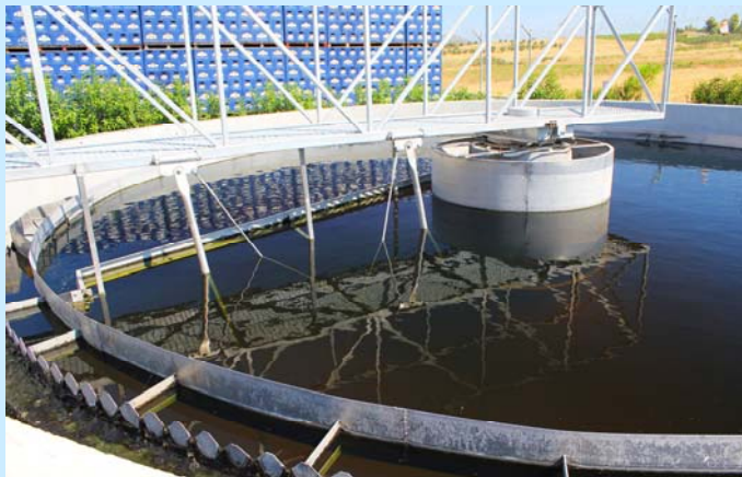
Final clarification tank
