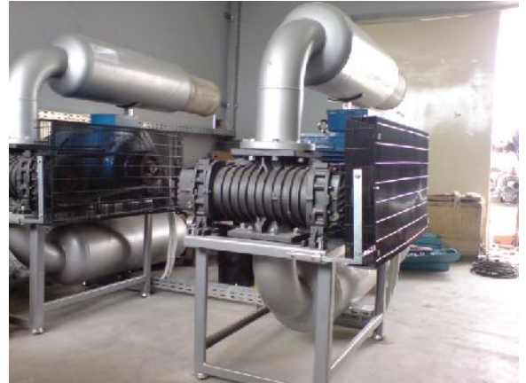
Equalization tank aeration blowers
