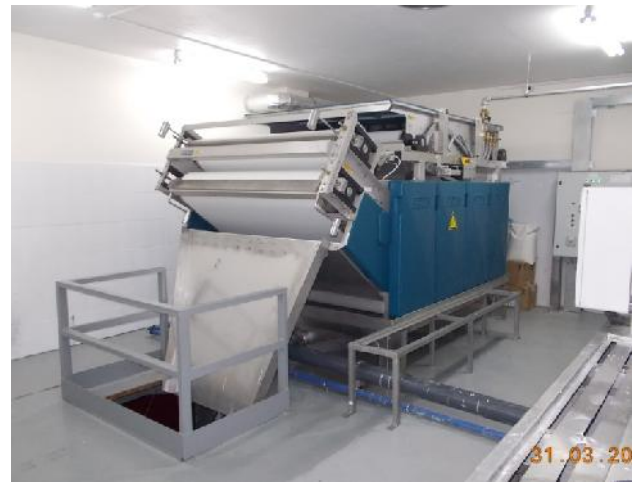
Sludge dewatering belt press
