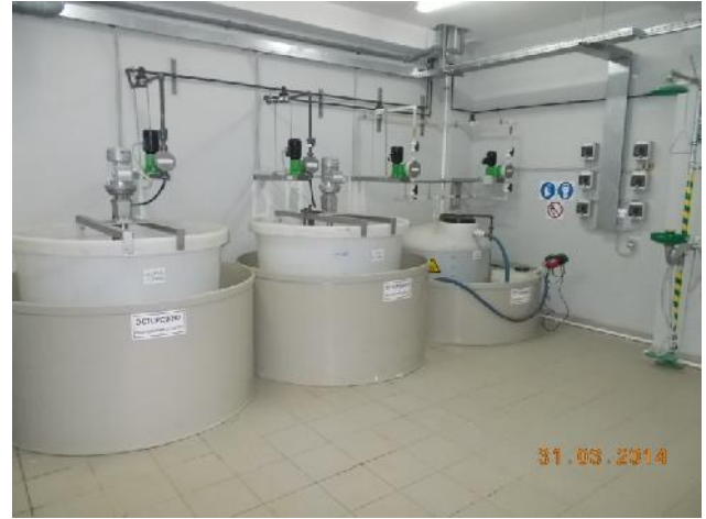
Chemical preparation and dosing
