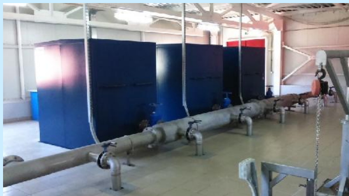
Blowers and air collector
