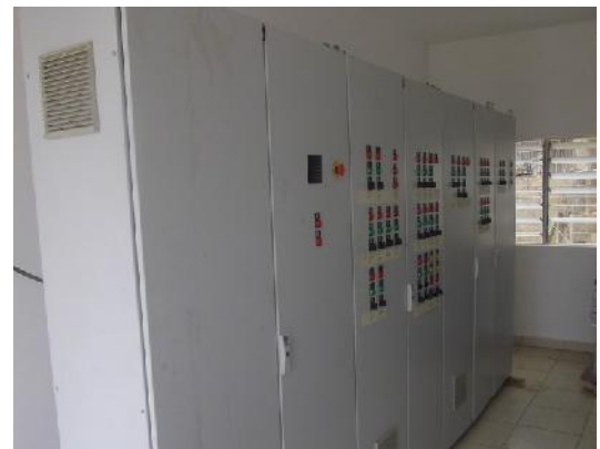
Main electrical panel
